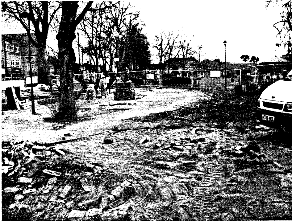
The direction of the passage was towards the Bingo Hall. This is the view away from the hole.
